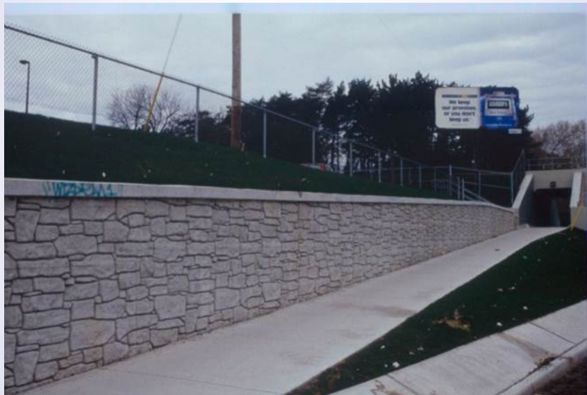
Patterned, textured concrete wall. Notice where the graffiti is!
